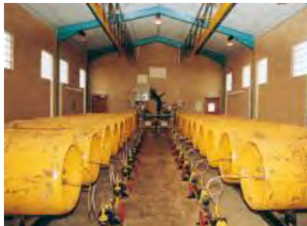
Figure 16: Typical large-scale chlorine gas disinfection system (Waterwise)
