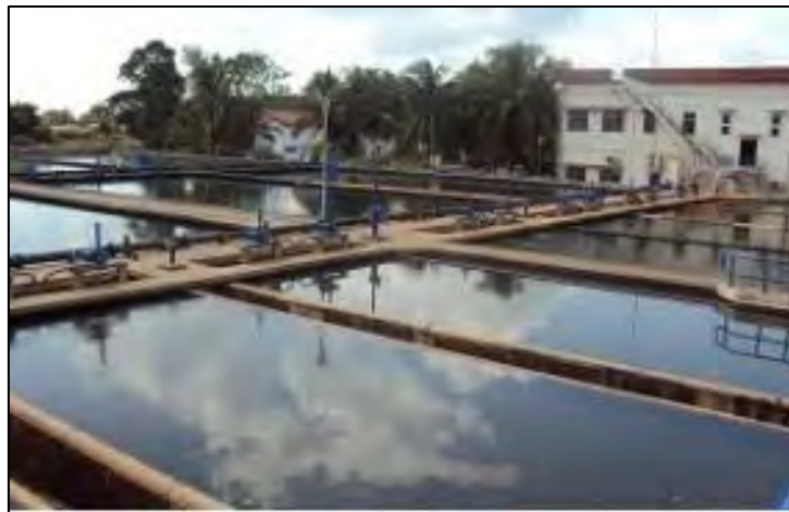
Figure 15: Typical rapid gravity sand filter plant (Nampapa Nakhoneluang)
