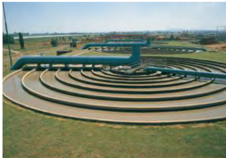
Figure 9: Typical circular static hydraulic flocculator (Rand Water – from Waterwise)
